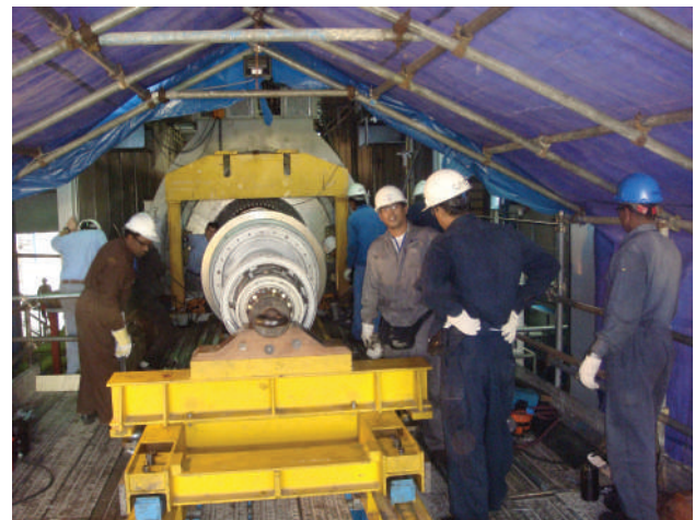
Meghnaghat Power Ltd.
